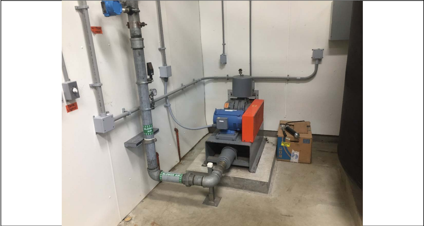
Backwash scour compressor.
