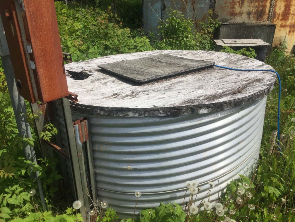
Pump basin to fill standpipe (note electrical cord running to heat trace).
