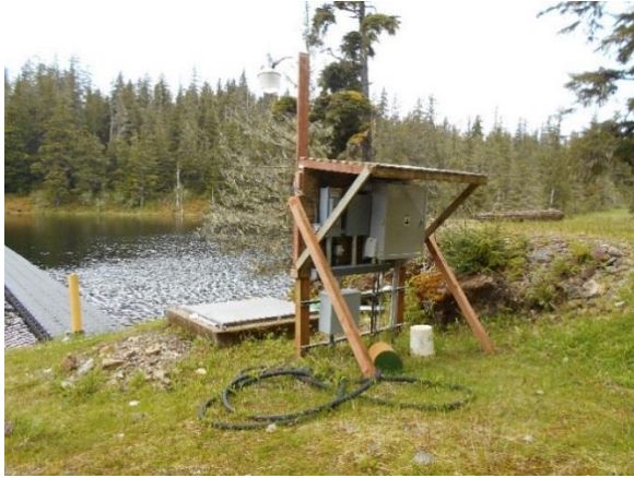
Figure 3.11: Water intake gallery near the Auk'tah Lake.
