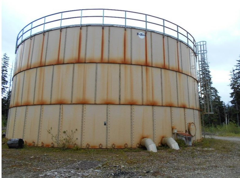
Figure 3.1: 500,000 gallon water storage tank in Angoon
