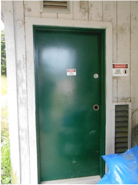
Figure 3.6: Generator Room door with no doorknob.
