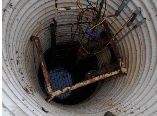
Figure 3.12: Water intake pumps in the gallery near Auk'tah Lake.
