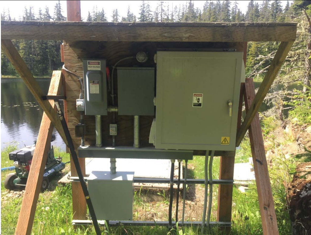
Pump controls center.
