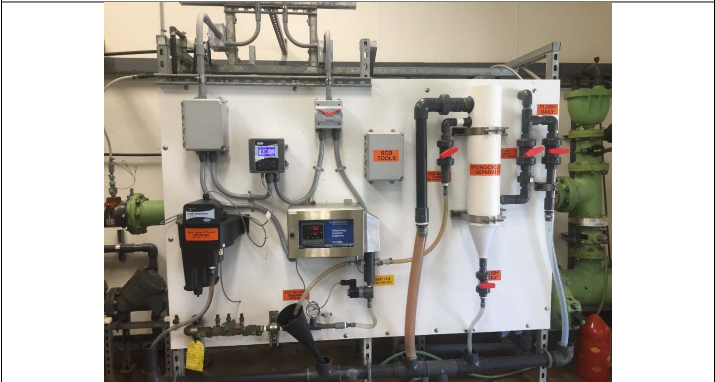
Streaming current detector and raw water turbidimeter.
