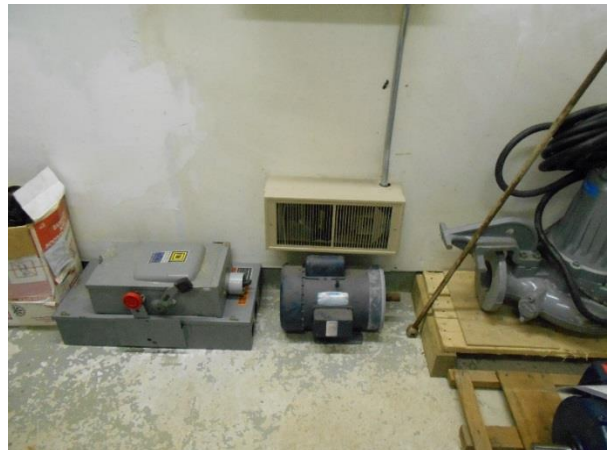
Figure 3.14: Electric heater in the generator room.
