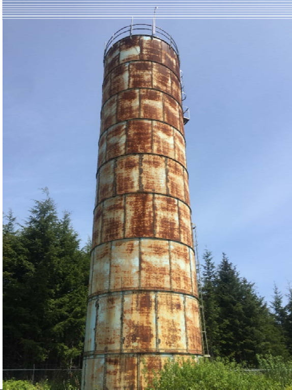
All tanks and standpipe showed rust streaking and evidence of leaks.
