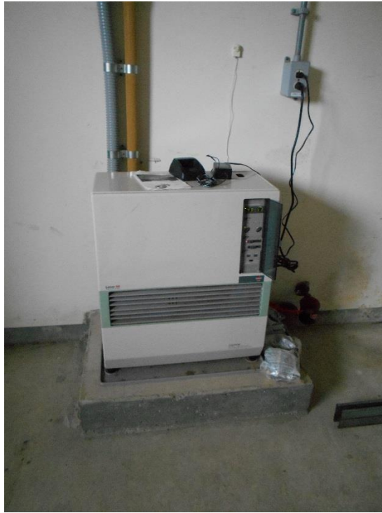
Figure 3.8: Toyotomi Laser 56 in the chemical room of the water treatment plant.
