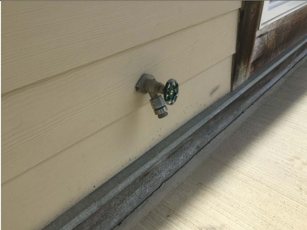
Vacuum breakers on hose bibs, typical at city offices, school and clinic.
