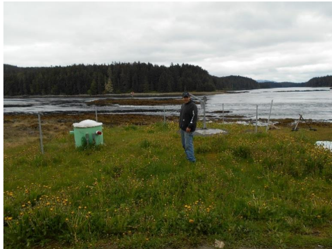
Figure 3.3: Kootznahoo lift station. This lift station is not in operation. Pictured is operator Danny Frederickson
