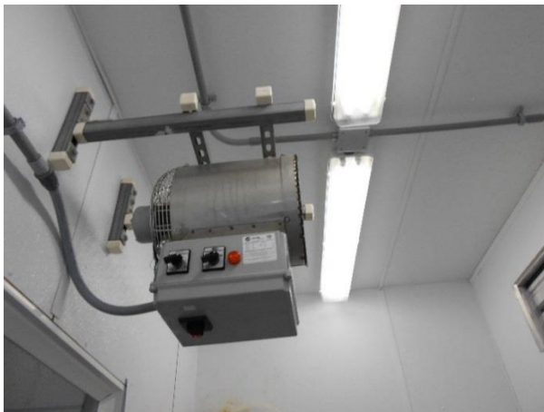
Figure 3.13: Electric heater in the chlorine room.
