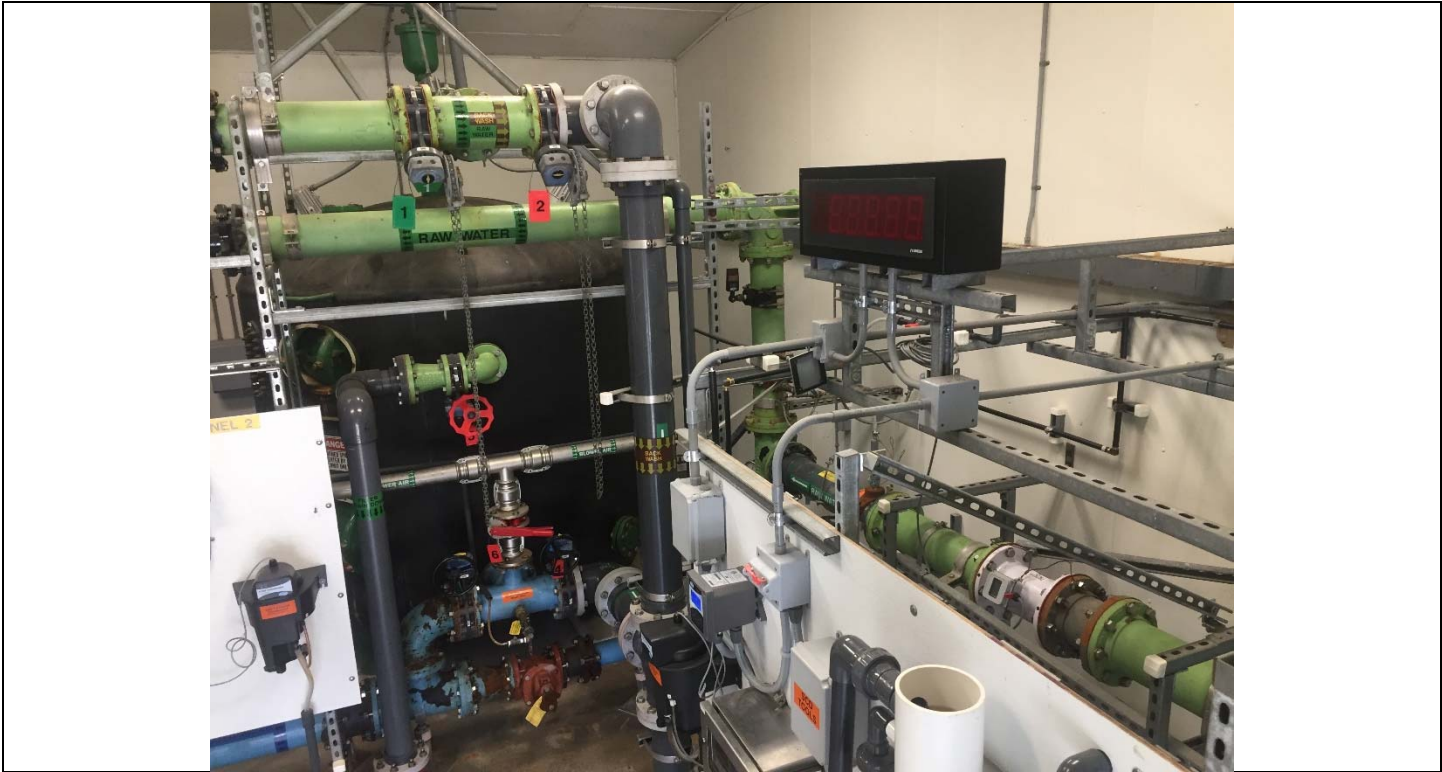
Coagulant mixing structure and Filter #1 in background.
