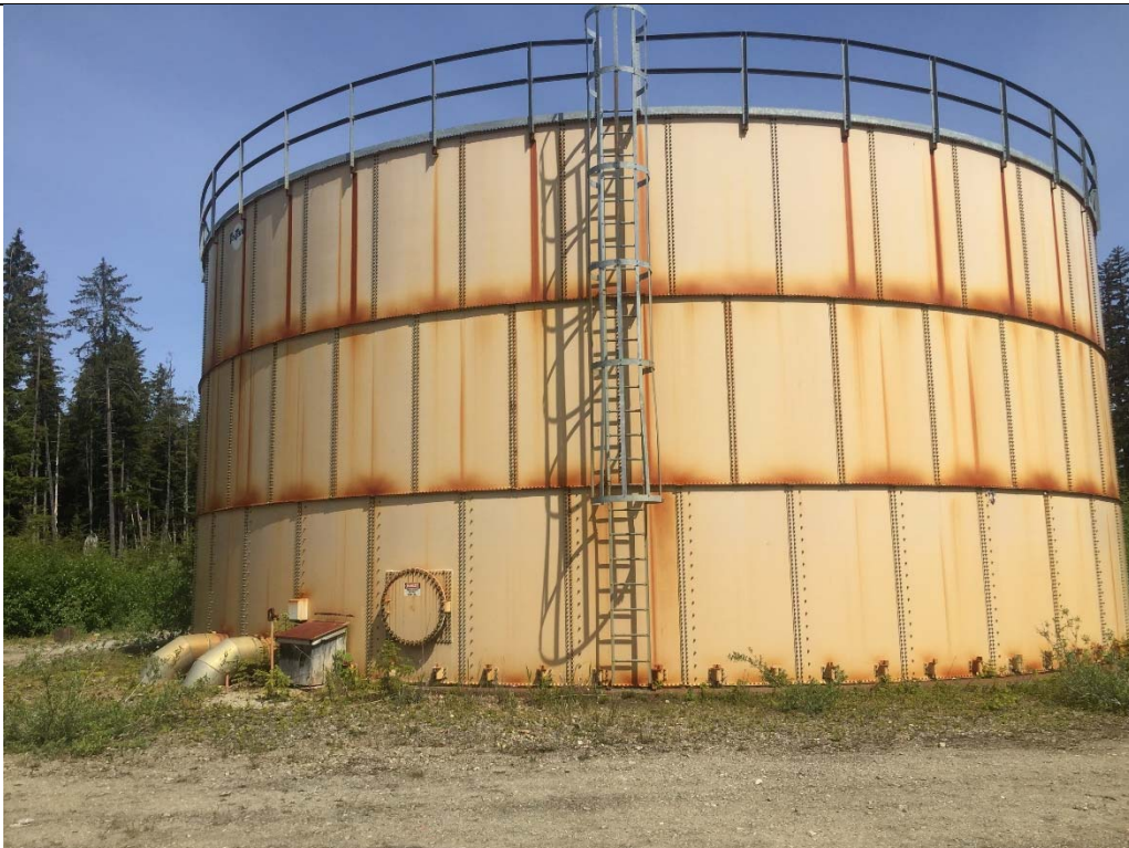
500,000 gallon finished water storage/contact tank.
