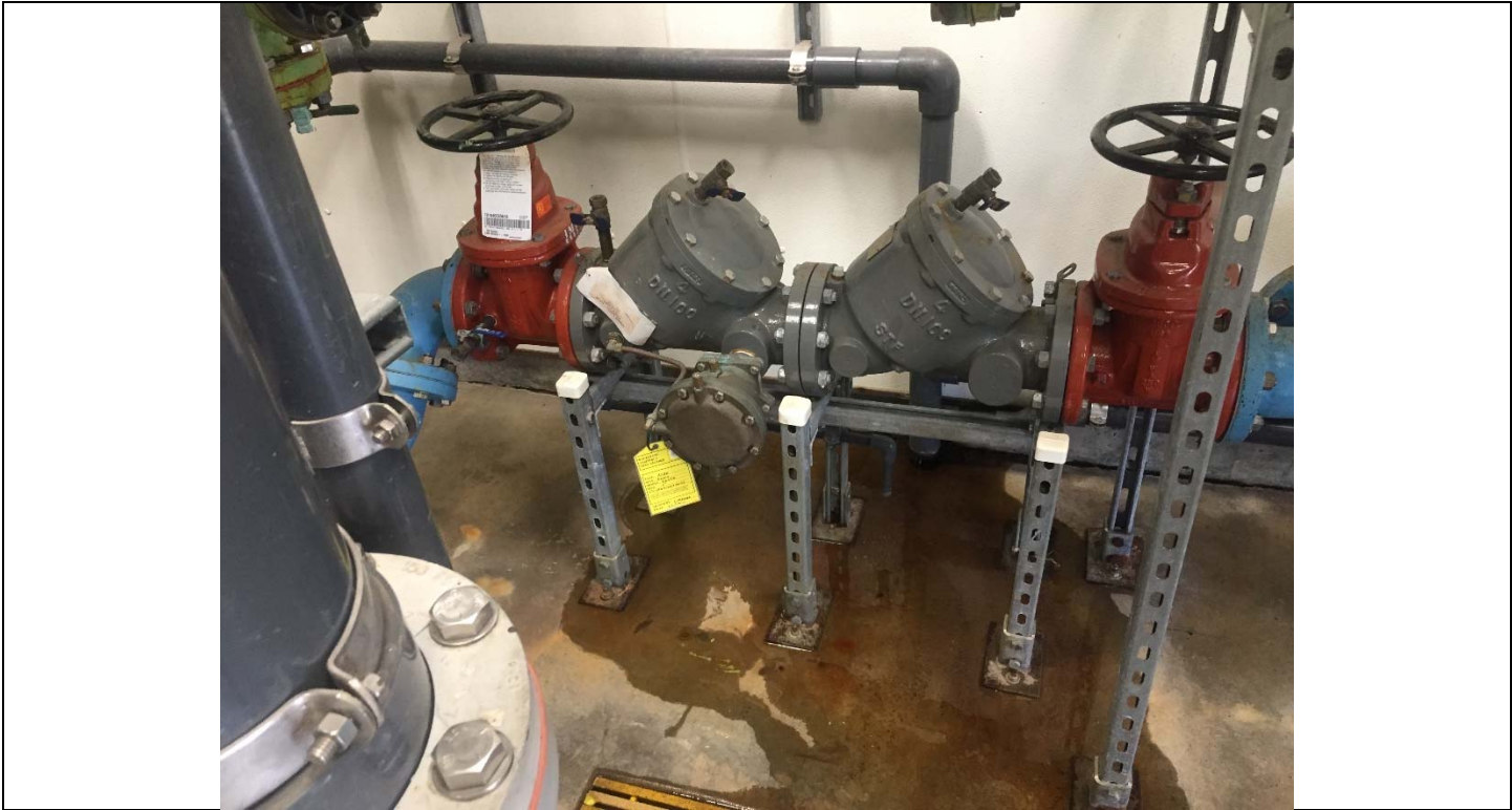
Backwash backflow prevention device.
