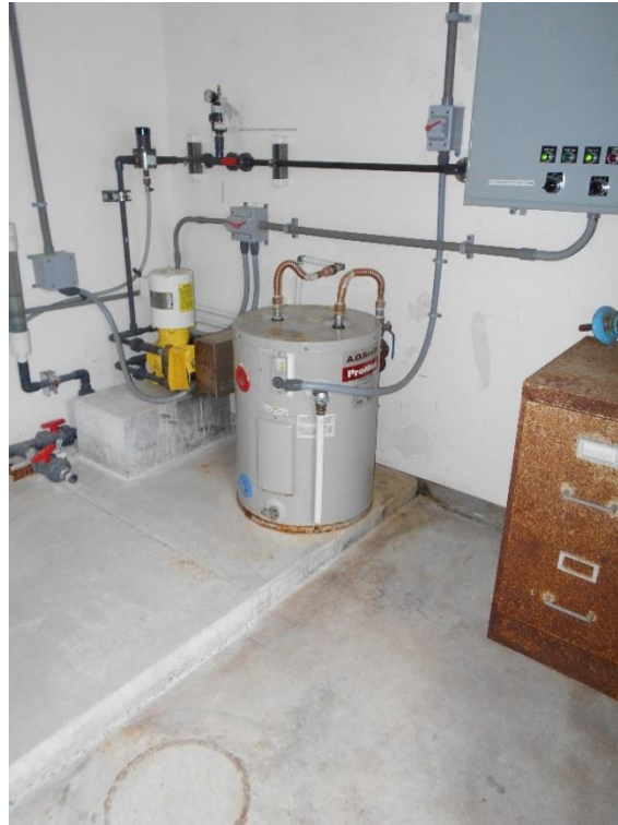
Figure 3.10: Electric hot water heater in the water treatment plant.
