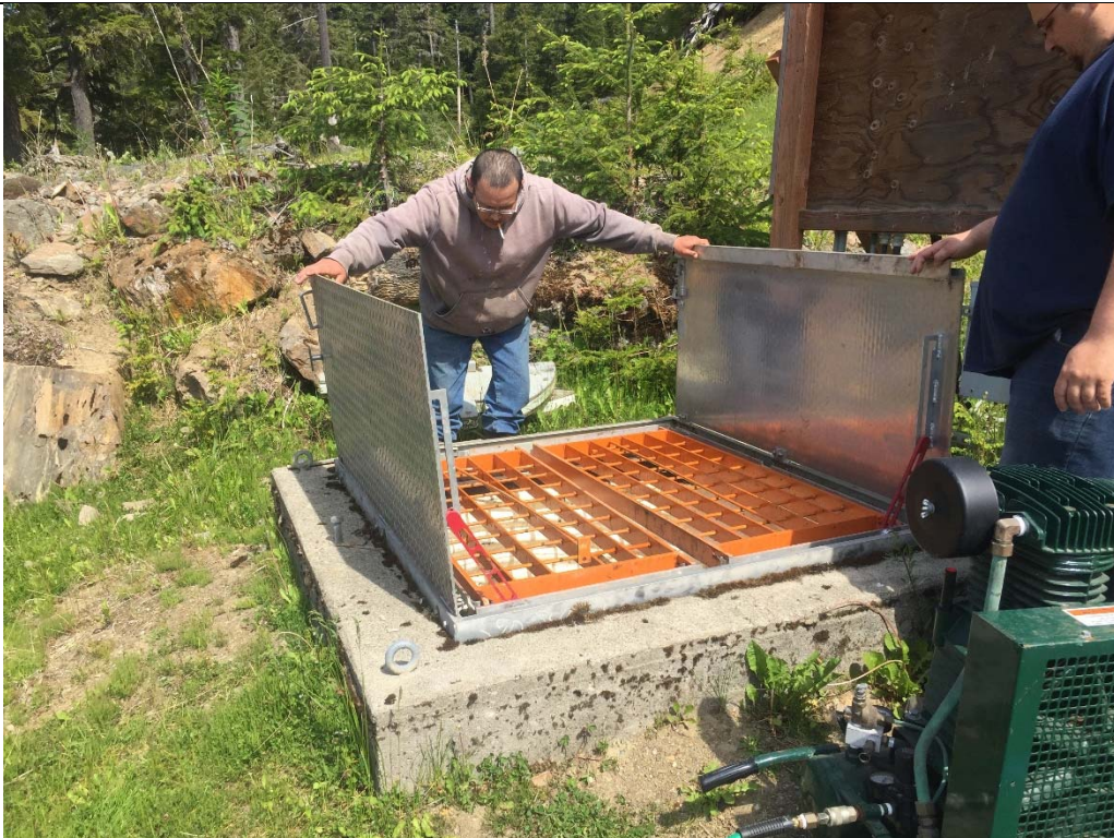
Raw water wet well with submersible pumps.
