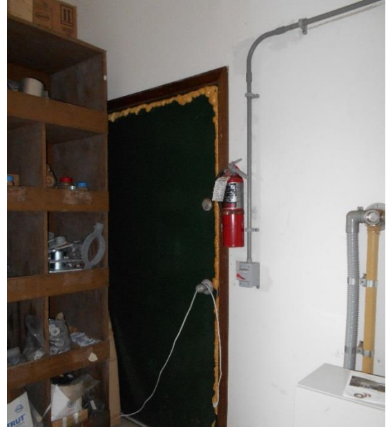
Figure 3.7: Chemical Room door with foam insulation sealing the spaces around the door frame.
