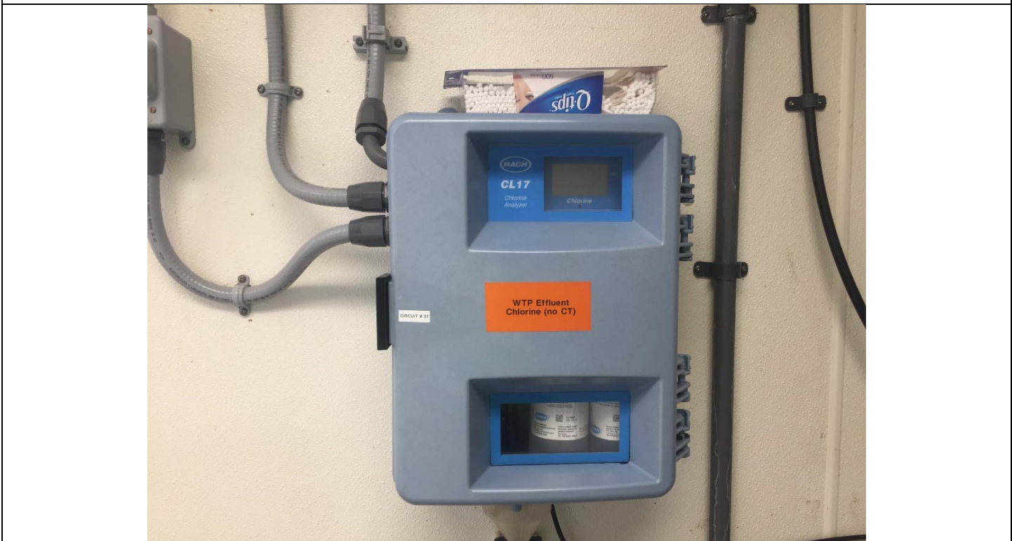
Finished water chlorimeter, out of service but the parts to put it back in service had arrived.
