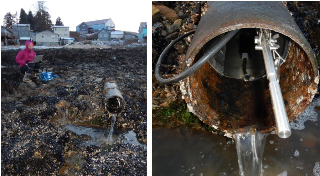
Figure 1: Flow Monitoring for Kootznahoo Lift Station
