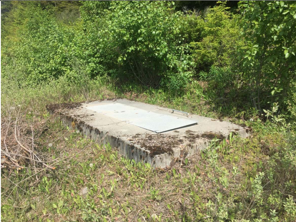
Pressure reducer vault between first storage tank and town.
