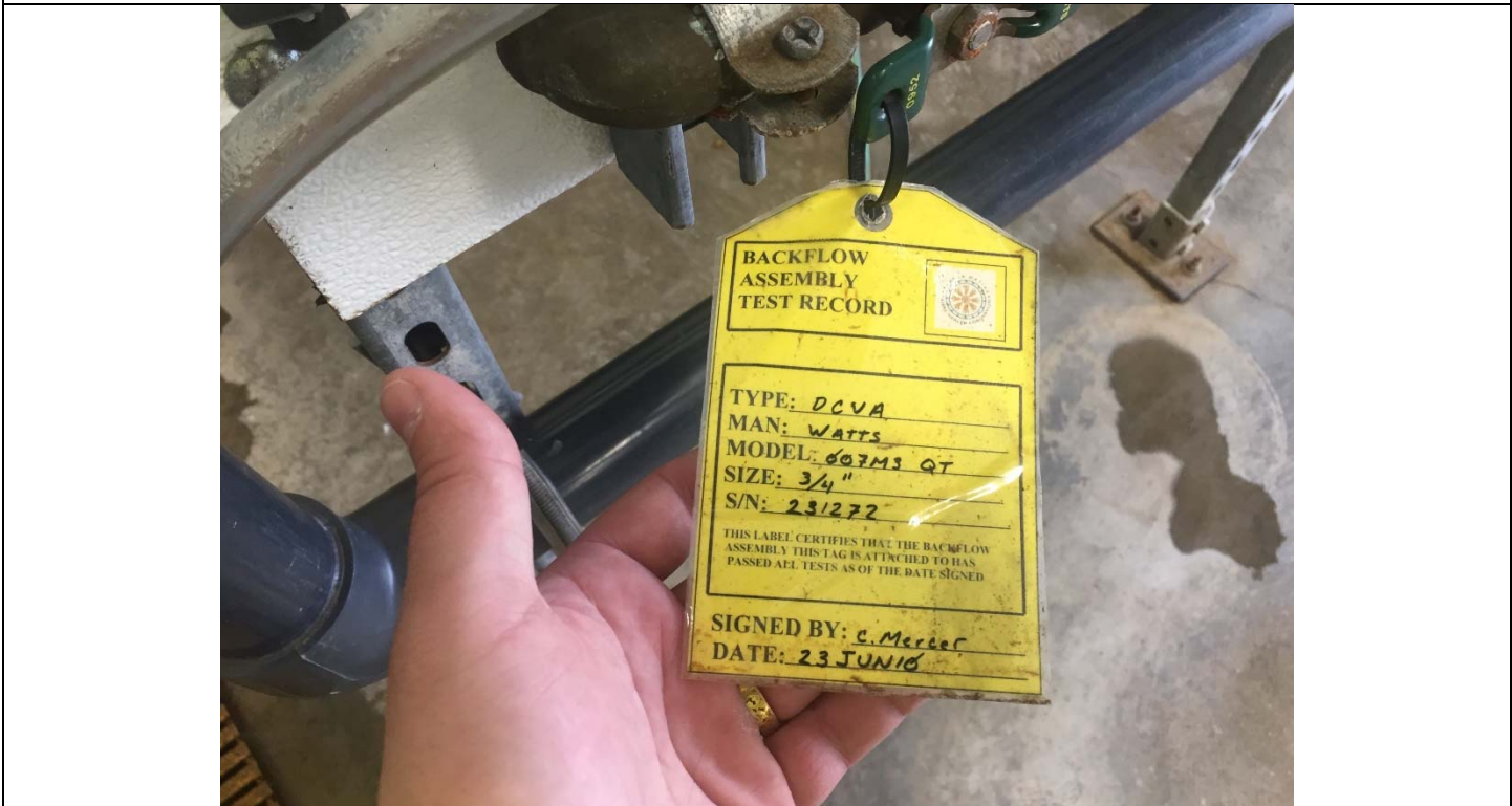
Backflow preventers all appear to have not been tested since installation.
