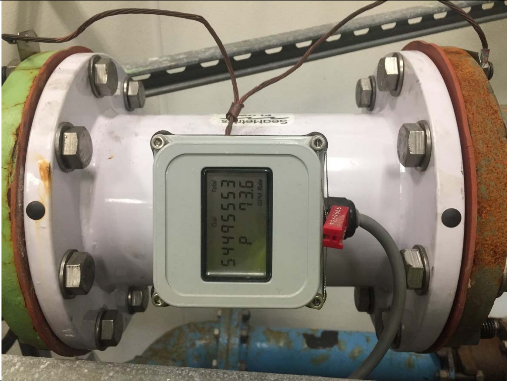
Raw water flow meter.
