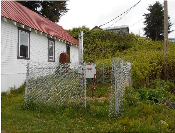
Figure 3.2: Downtown lift station on Anya Street
