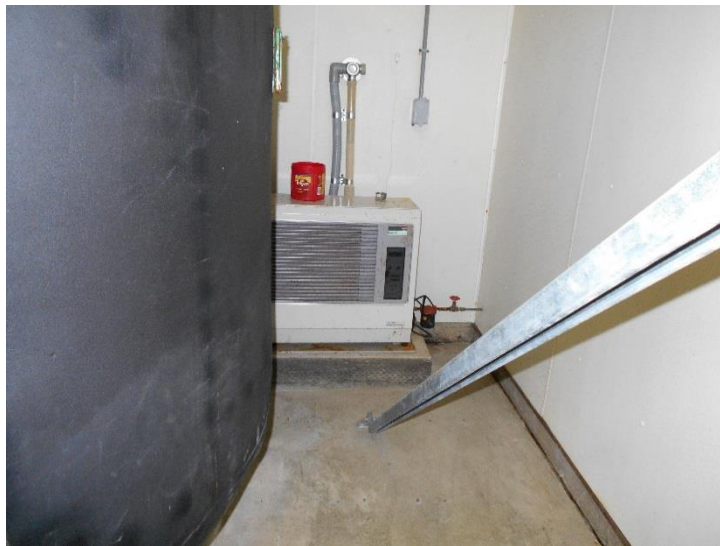
Figure 3.9: Toyotomi Laser 73 in the process room of the water treatment plant. This unit is not used.
