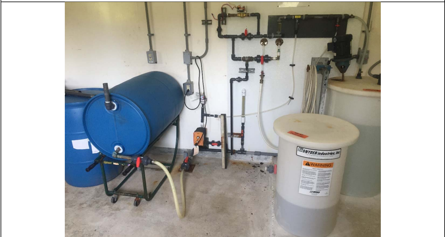
Polymer supply system.
